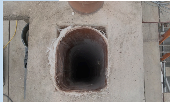
The lined duct.
